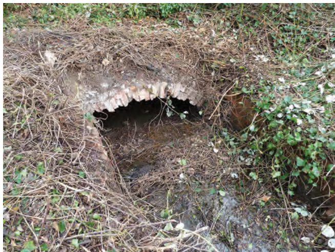
In 1991 the shallow Hollingwood Common Tunnel south of the 1890s Chesterfield Canal deviation was excavated.
